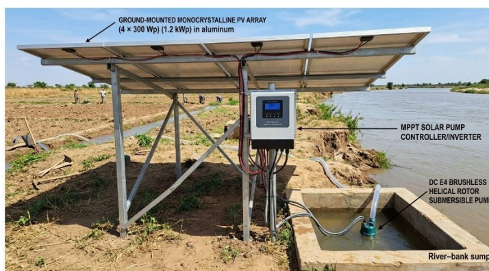
Figure 1. Field setup of the solar PV pumping system
